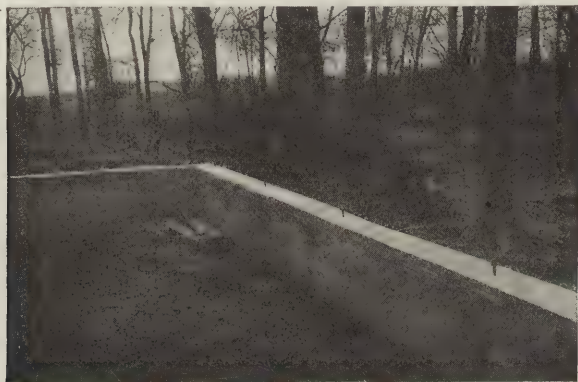
FIG. 13.—Foundation wall for a small shed, showing bolts for attaching the wooden sill to the concrete foundation.
